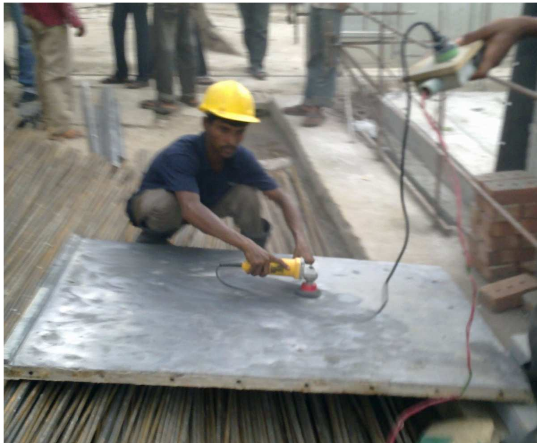
Shutter Brushing without Eye protection and hand-gloves Eye damage
