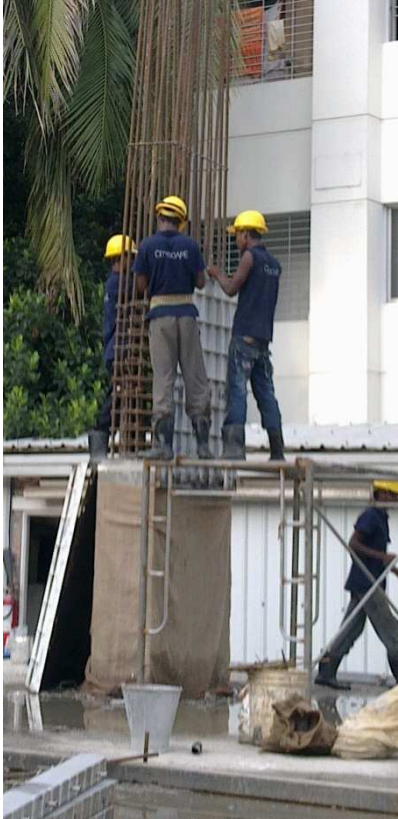
Improper Scaffolding, No Safety Belt Danger of falling
